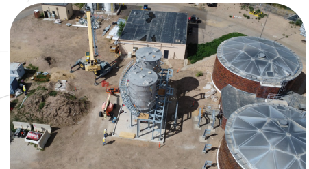
Phosphorus Reactor Tanks
