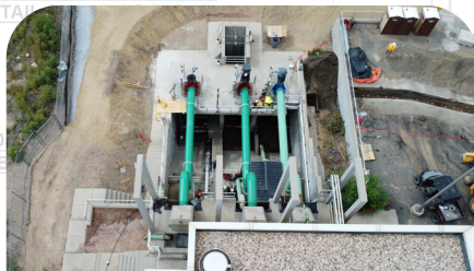
Influent Pumps & Piping
