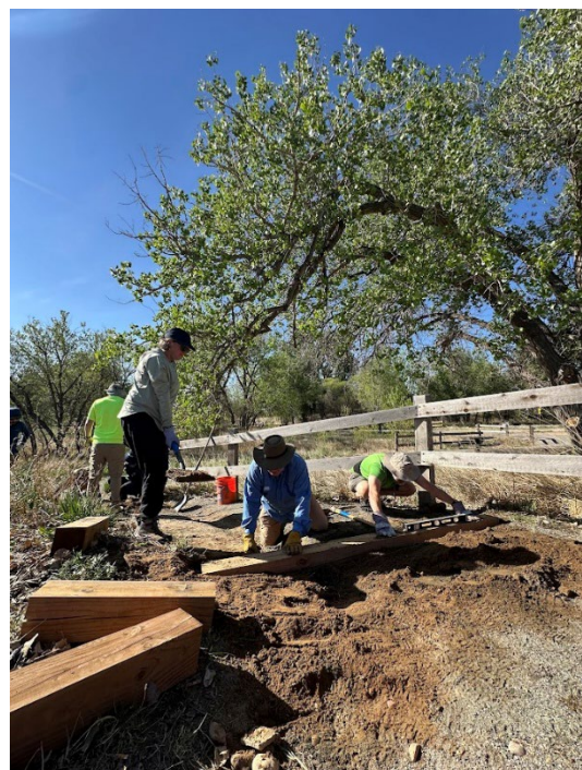
Volunteers construct trail stairs at McCloskey Natural Area as part of a volunteer project day.
