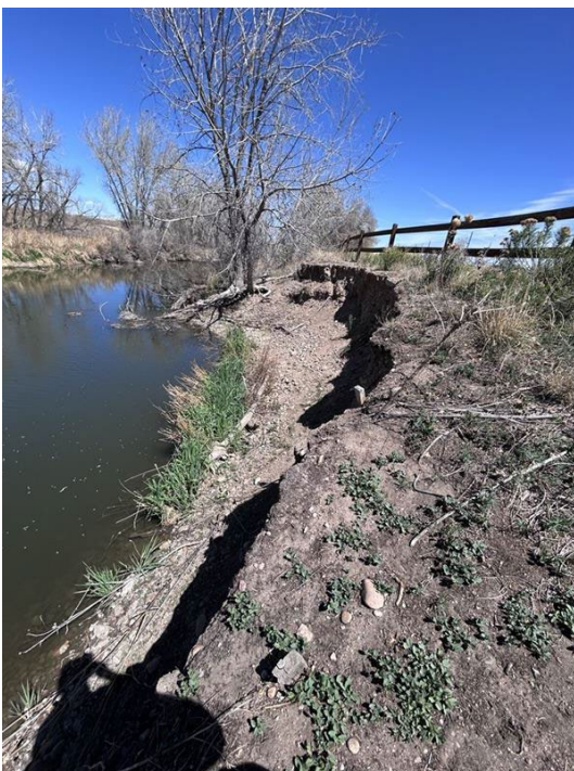
A new erosion area along the Poudre Trail, just north of the Rover Run Dog Park. Design will begin in 2026 to make emergency repairs.
