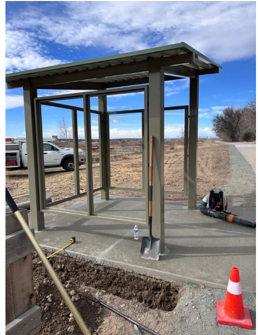
A new port-a-let enclosure is installed along the Poudre Trail at Poudre Ponds. This project is funded by Fishing is Fun and Great Outdoors
