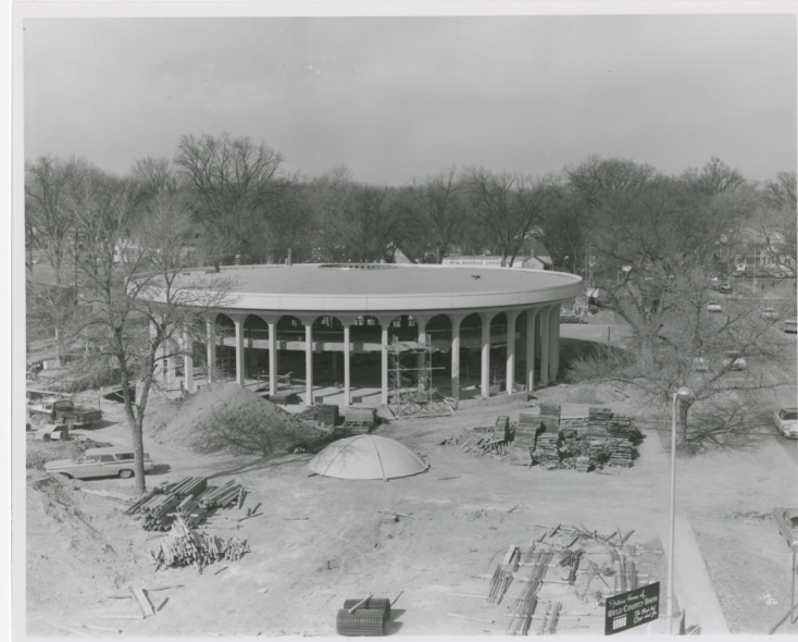
Below: Construction of Weld County Bank, 1000 10 th Street, 1967-68, photographer: Kadlecek Studios. Credit: 1992.75.0439, City of Greeley Museums, Lew Dakan Collection.
