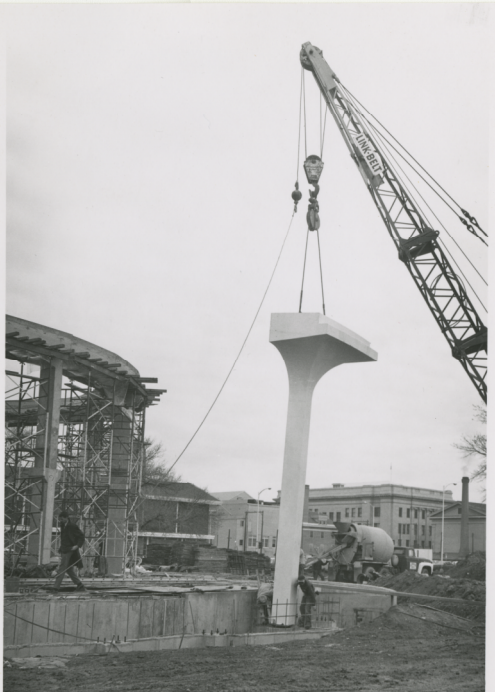
Construction of Weld County Bank, 1000 10 th Street, 1967-68, photographer: Lew Dakan. Credit: 1992.75.0554, City of Greeley Museums, Lew Dakan Collection.
