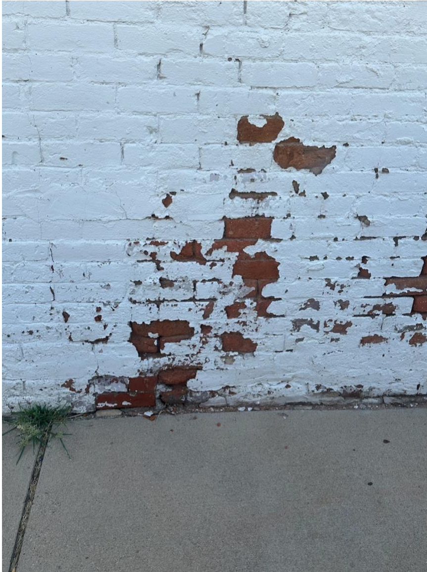
View of existing painted brick on west side of building. Paint is chipped and will be repainted. ( View of photo is facing east )
