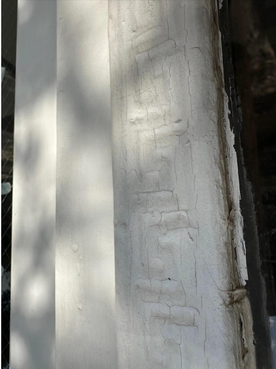
Close-up of existing Greek key design that surrounds the windows. It has many layers of paint that are cracking in the sections of the material that still remain. ( View of photo is facing west )
