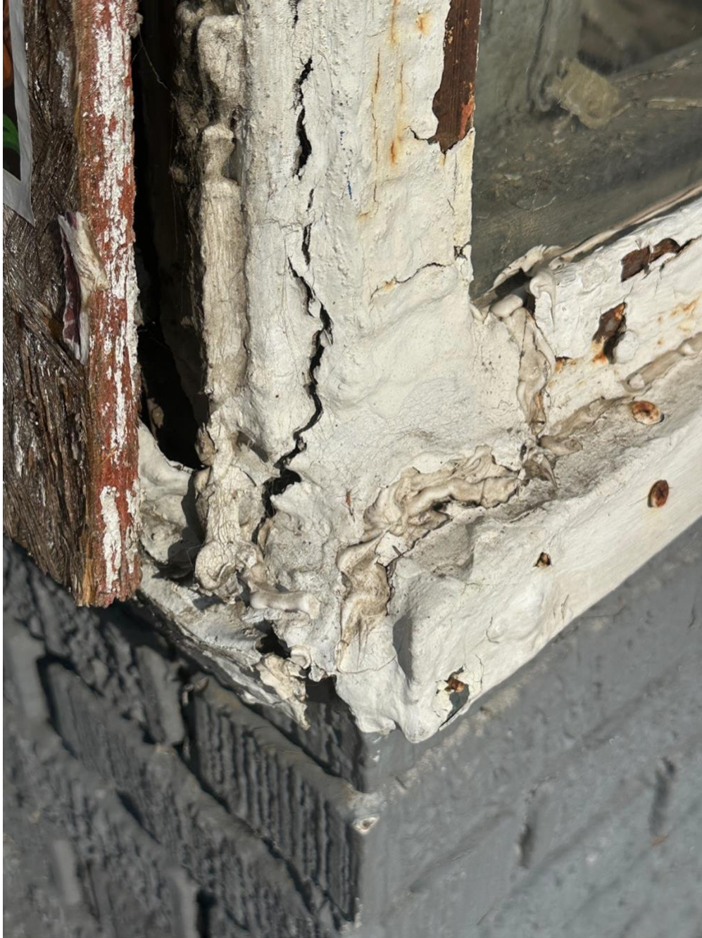
Close-up photo of the window base on the SE corner of the building. Many layers of paint are decaying on the existing Greek key design and the window itself has come away from the building. ( View of photo is facing NW )
