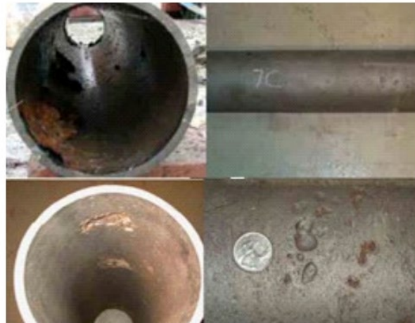
6" CI pipe with 10% measured loss
