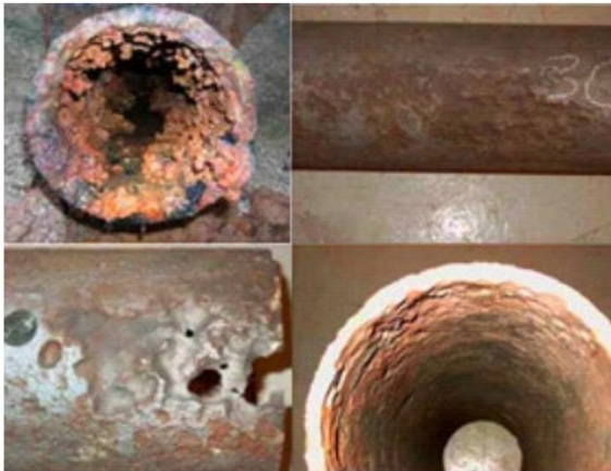
6" CI pipe with 47% measured loss
