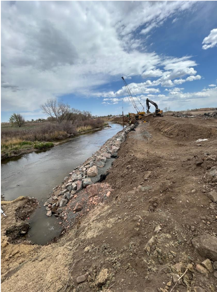
A crane places sheet pilings 16 feet deep in the southern riverbank of the Poudre River at Poudre Ponds, while crews follow behind to place 3-4 ft boulders above to construct the lower wall.
