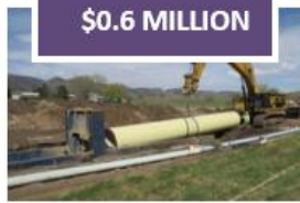
Bellvue Pipeline Goldhill Segment
