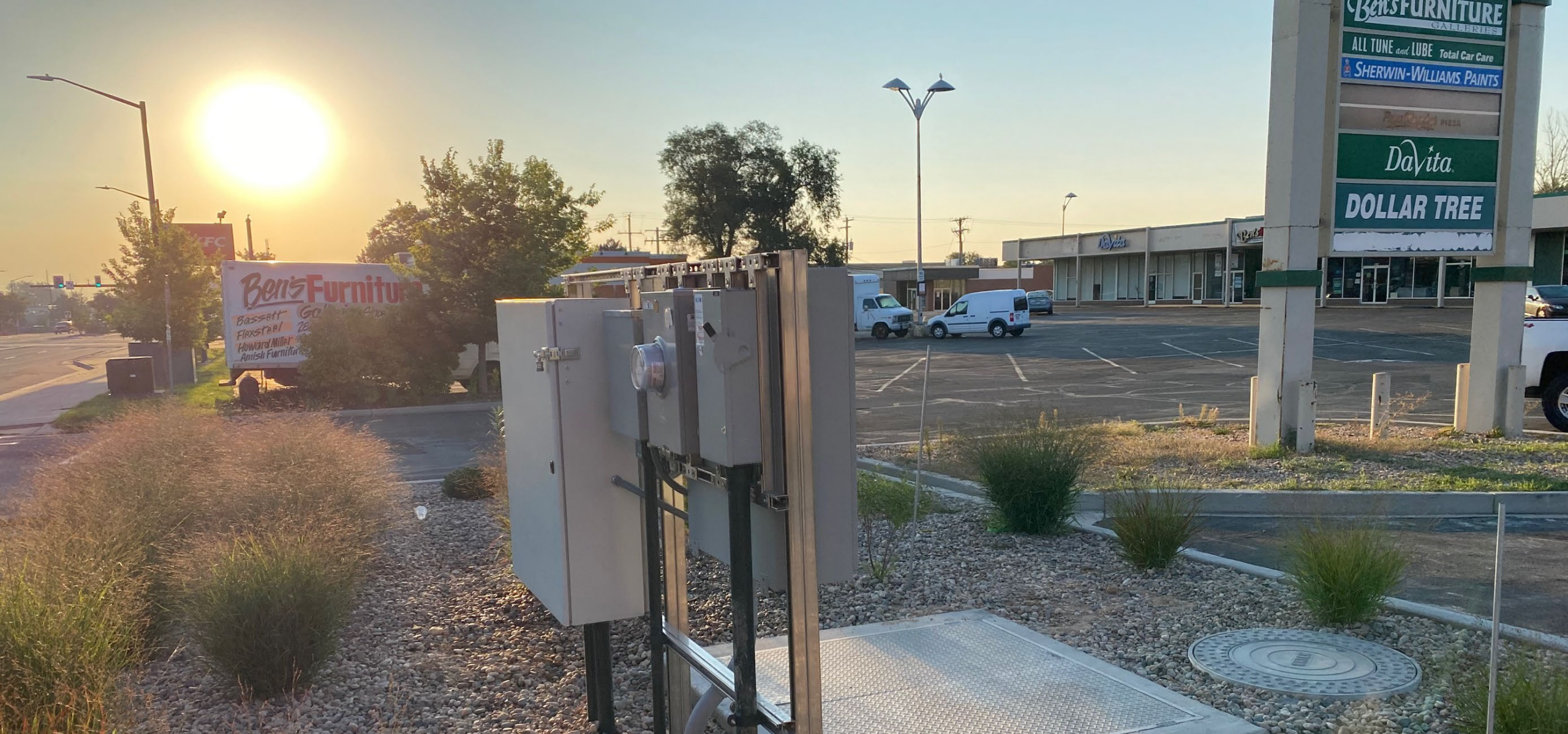
PRV 28 (10th Street)
