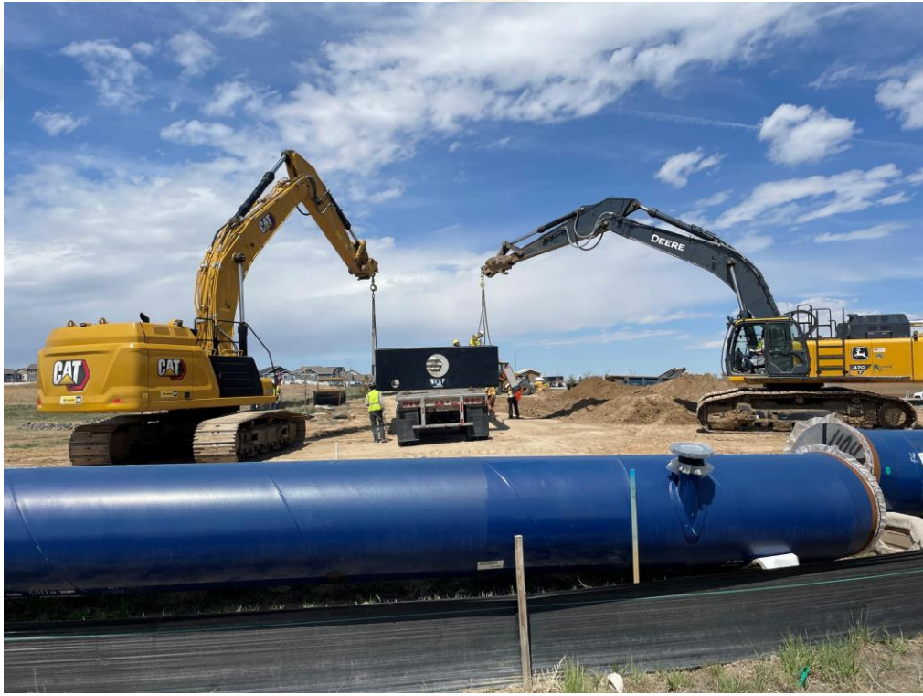
Unloading vault at Hwy 14 and CR 15
