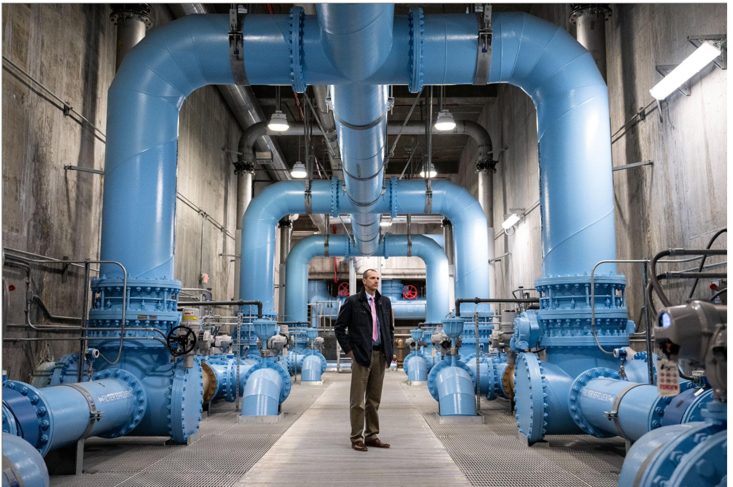
Brett Henry, executive director for infrastructure of Thornton, Colo., at the city's water treatment plant.
