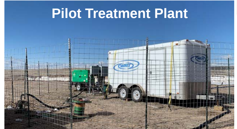
Ion Exchange Columns
