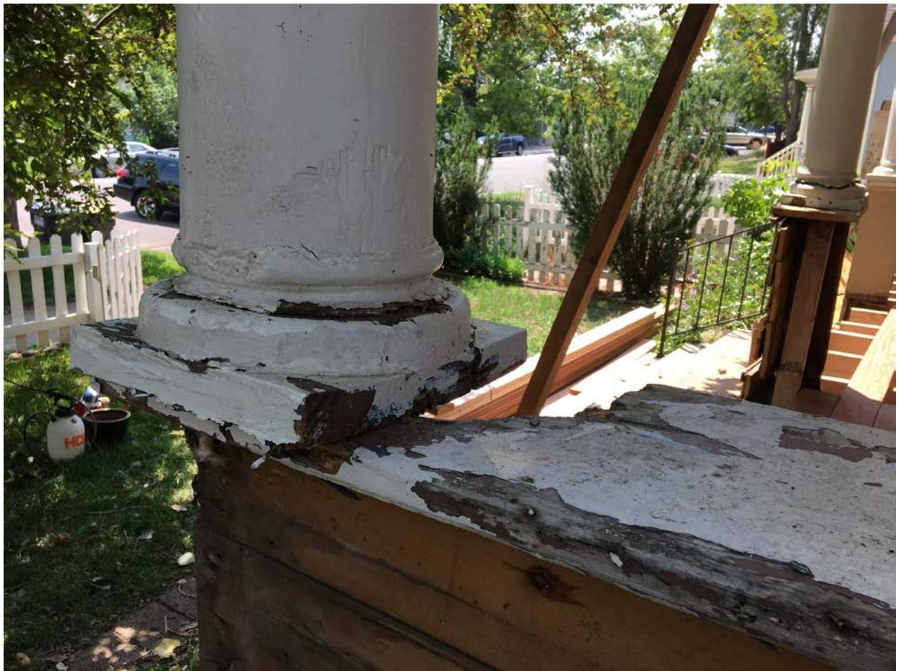
Severely deteriorated porch rail and column support
