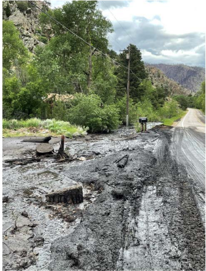
Photo 3. Sediment, ash & debris from stream overtopping HWY 14 on June 25, 2021
